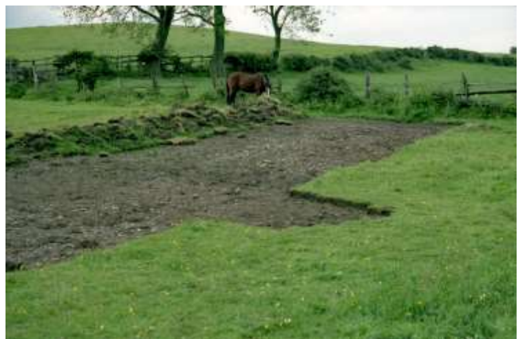
Work begins on the car park area at the Flamsteed Observatory site.
